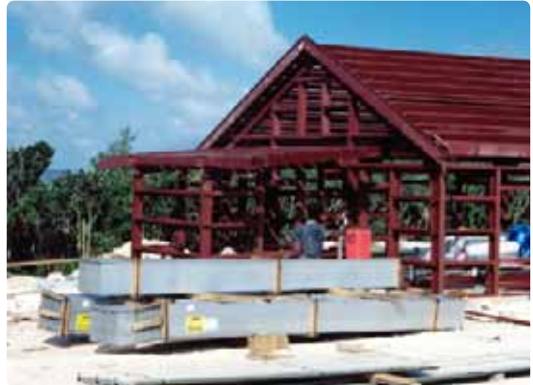
Prefabricated Building for Utilities
