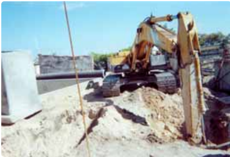
Storm Water Management Systems
