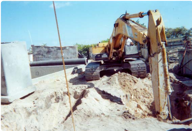
Storm Water Management SYstems
