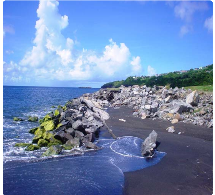
Post-Storm Revetment Conditions
