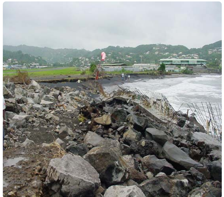
Post-Storm Revetment Conditions
