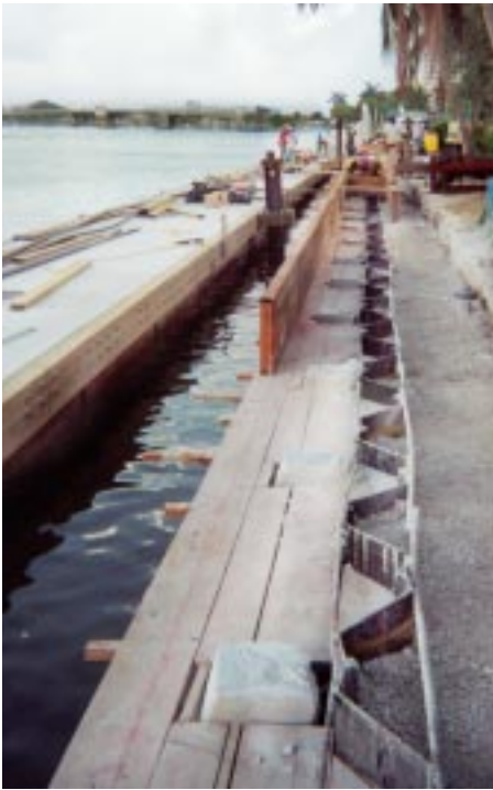
Replacement steel sheet pile bulkhead under construction, Bahia Mar Yachting Center, Ft. Lauderdale, Florida
