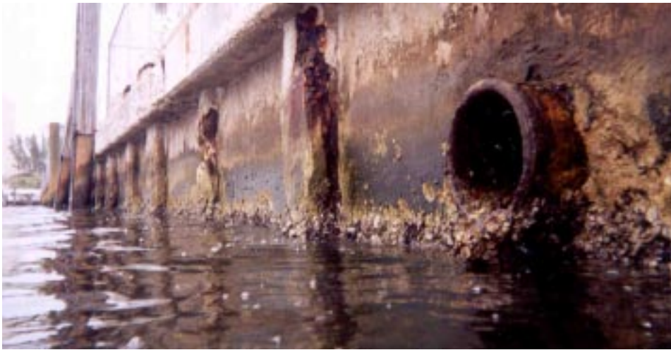
Deteriorated concrete pile/panel bulkhead. Note the storm sewer outfall through the bulkhead.
