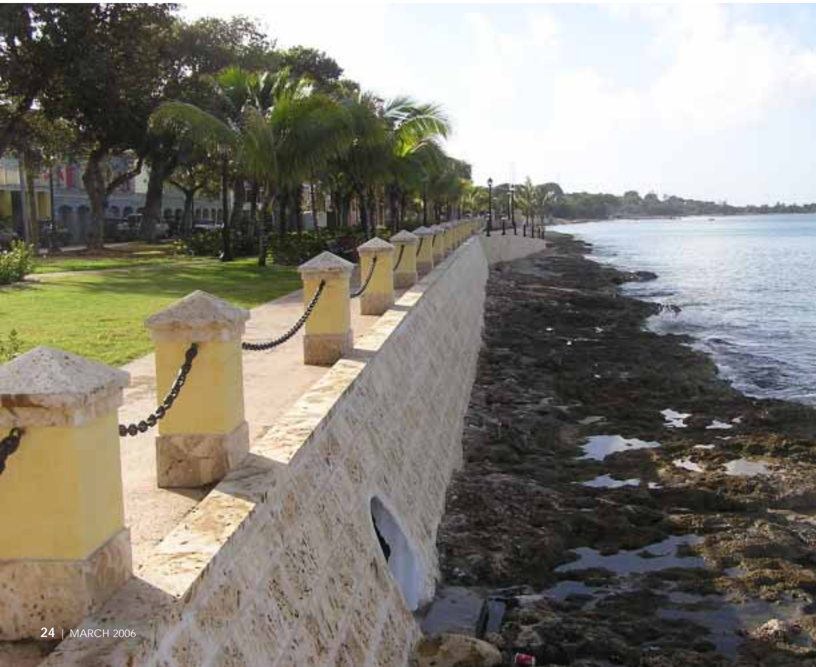
Improvements to the shoreline include a new, tiled seawall for Veterans Park, with new concrete bollards with limestone caps along the top.
