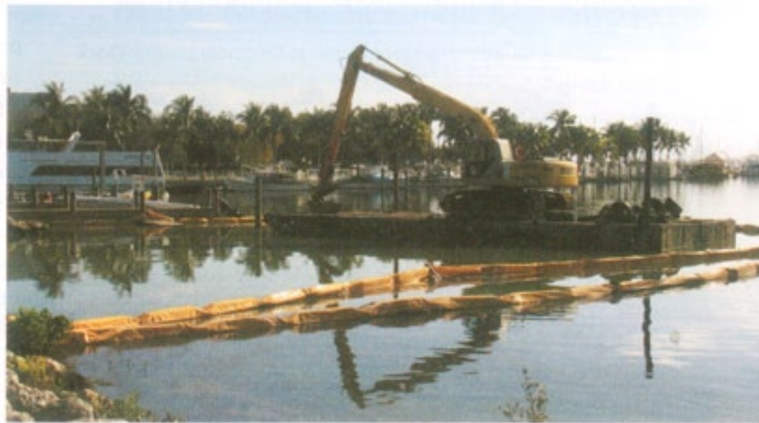
The $1.4 million dredging project at Dinner Key Marina in Miami began at Seminole Dinghy Dock & Boat Ramp. A mechanical dredge will remove 9,000 cubic yards of sediment.
