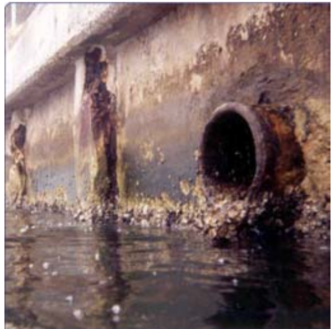
Deteriorated concrete pile/panel bulkhead. Note storm sewer outfall through bulkhead.
