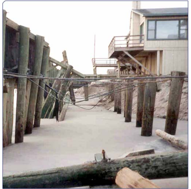
Damaged timber seawall
