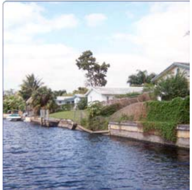
Failed bulkhead due to inadequate embedment of wall.
