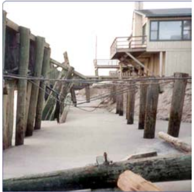
Damaged timber seawall
